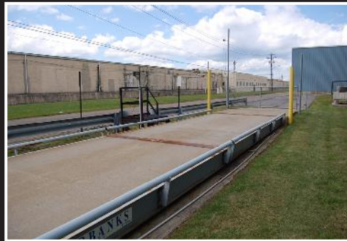
Fairbanks truck weigh scale; 130' x 69', monitored by camera, (2) exterior displays, (8) load cells
