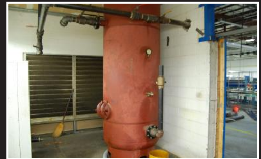
Air receiving tank; 1994 vintage, 150 psi rating, 9' x 40" diameter
