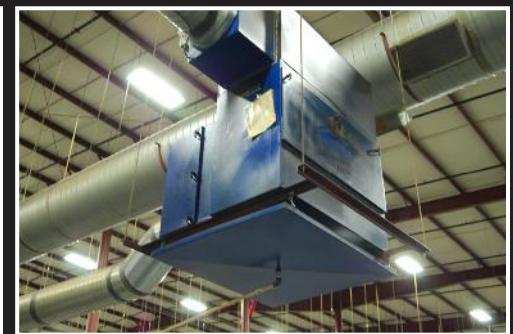
Clark air mist collector/ filtration unit (40+ through out facility)
