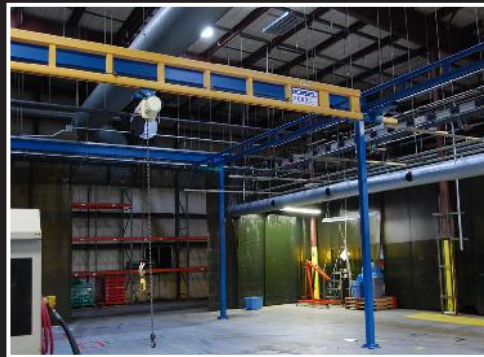
Gorbel 2000 klb capacity free standing hoist; Coffing JLC 1 ton hoist, approximate 34' span, approximate 57' runway, 10' hook to floor
