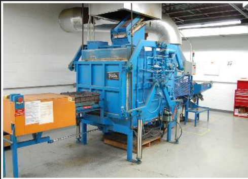
Refractory Maintenance Corp heat treat furnace; natural gas fired, Honeywell controls and components, air accuated doors
