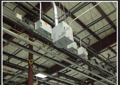
hundreds of feet of bus bar and plugs
