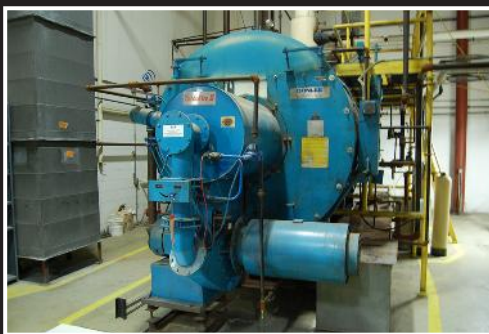
Donlee Technologies YSL-300-N200-285 package boiler; 1997 vintage, firing rate 12562 cfh, rated steam capacity 10.043.000, max working pressure = H2O @ 30 and steam @ 15, serial 97-204-84 H-12549
