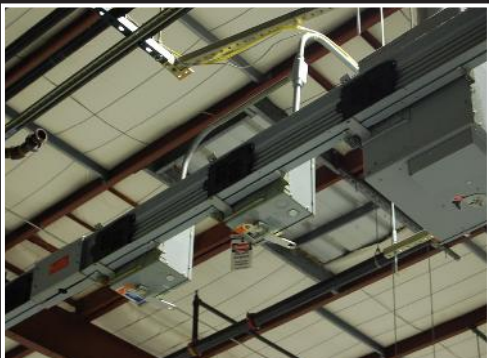
hundreds of feet of bus bar and plugs
