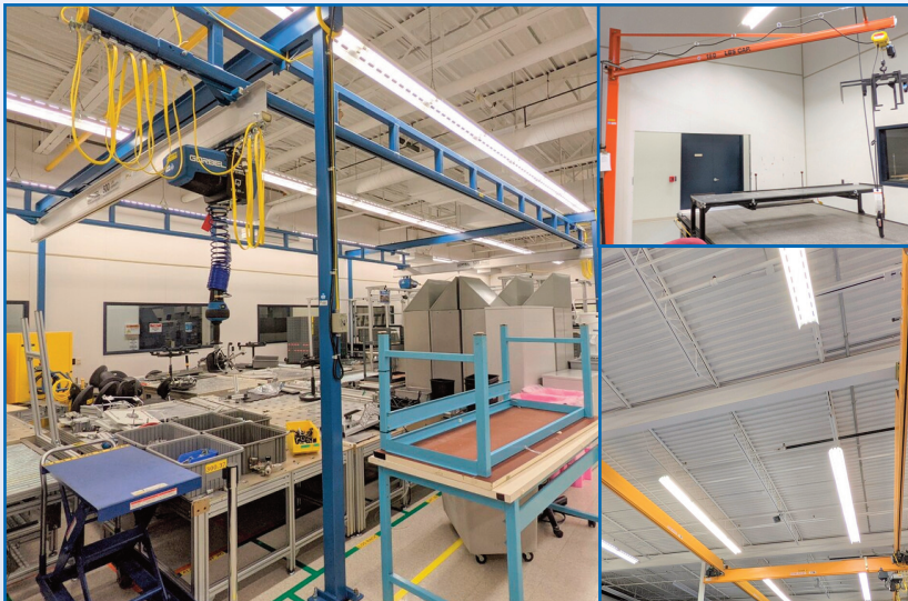
PARTIAL VIEW OF FREE STANDING, OVERHEAD AND JIB CRANES
