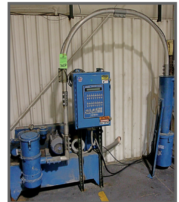
2002 NOVATEC MCS-216 MATERIAL DISTRIBUTION SYSTEM
