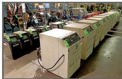
VIEW OF TEMPERATURE CONTROLLERS
