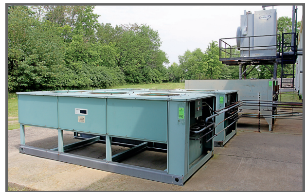
VIEW OF WATER SYSTEMS
