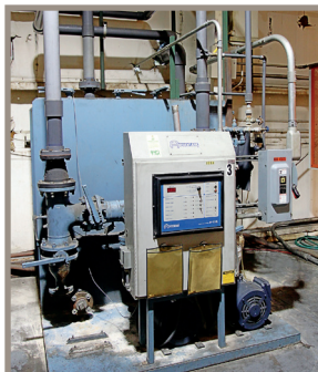
ADVANTAGE PTS-800-3P CHILLER
