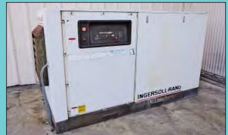
50 HP Ingersoll Rand Model SSR-XFE50 Cabinet Enclosed Rotary Screw Air Compressor
