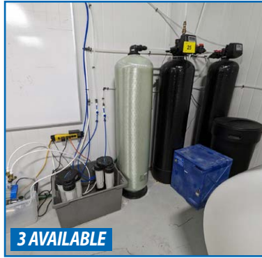
PARTIAL VIEW OF REVERSE OSMOSIS SYSTEMS
