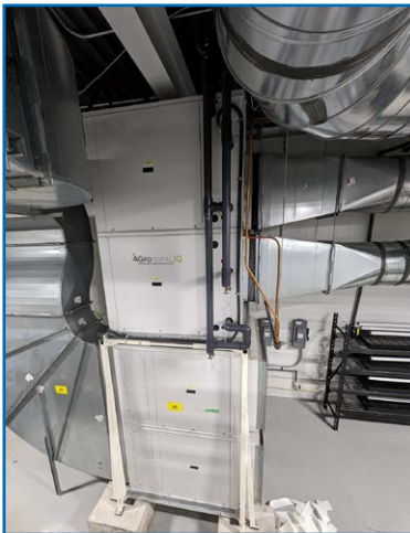
AGRONOMIC IQ INTELLIGENT GROW ROOM HVAC SYSTEMS
