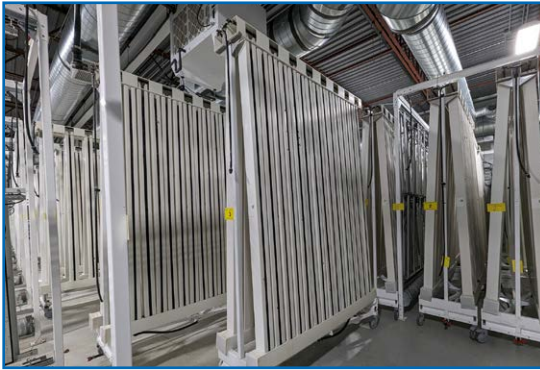
PARTIAL VIEW OF CUSTOM BUILT VERTICAL FARMING / GROWING CARTS
