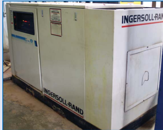
INGERSOLL RAND RS AIR COMPRESSOR
