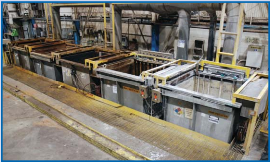
(5) HT NITAL ETCH EQUIPMENT DIP TANKS
