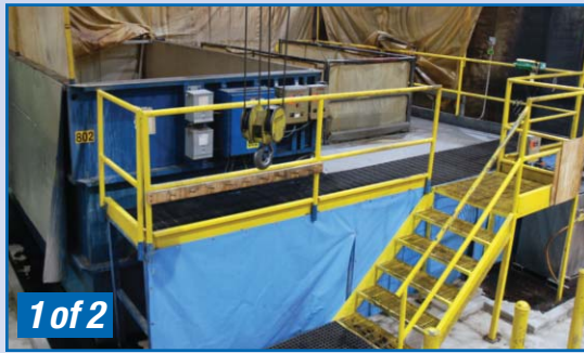
(4) AQUEOUS DEGREASE HOT WATER RINSE TANKS
