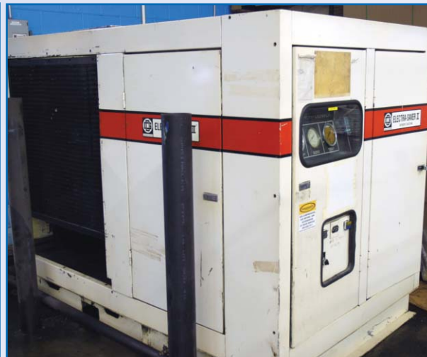
GARDNER DENVER 75 HP COMPRESSOR
