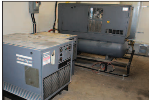
View of Rotary Screw Air Compressors
