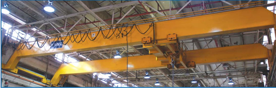
KONE 25 TON X 65' BRIDGE CRANE
