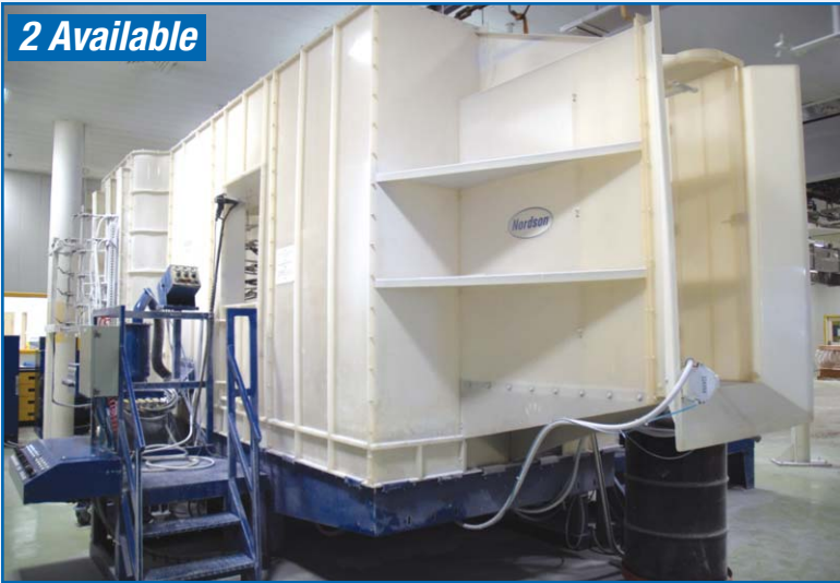
NORDSON EXCEL 2000 MODEL 2002S ELECTROSTATIC POWDER COAT PAINT BOOTH SYSTEMS
