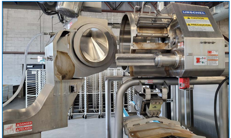
PARTIAL VIEW OF WASH LINE
