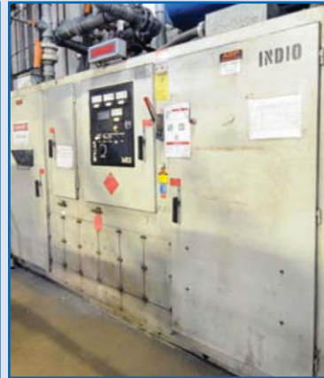
PILLAR MK8 CORELESS INDUCTION MELTING FURNACE CONTROLS
