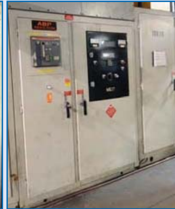
ABP MK17 CORELESS INDUCTION MELTING FURNACE CONTROLS
