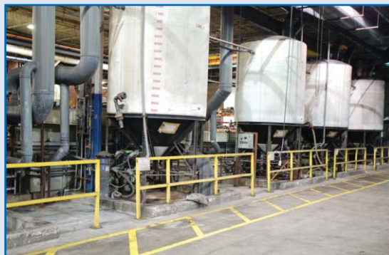
PARTIAL VIEW OF TANKS
