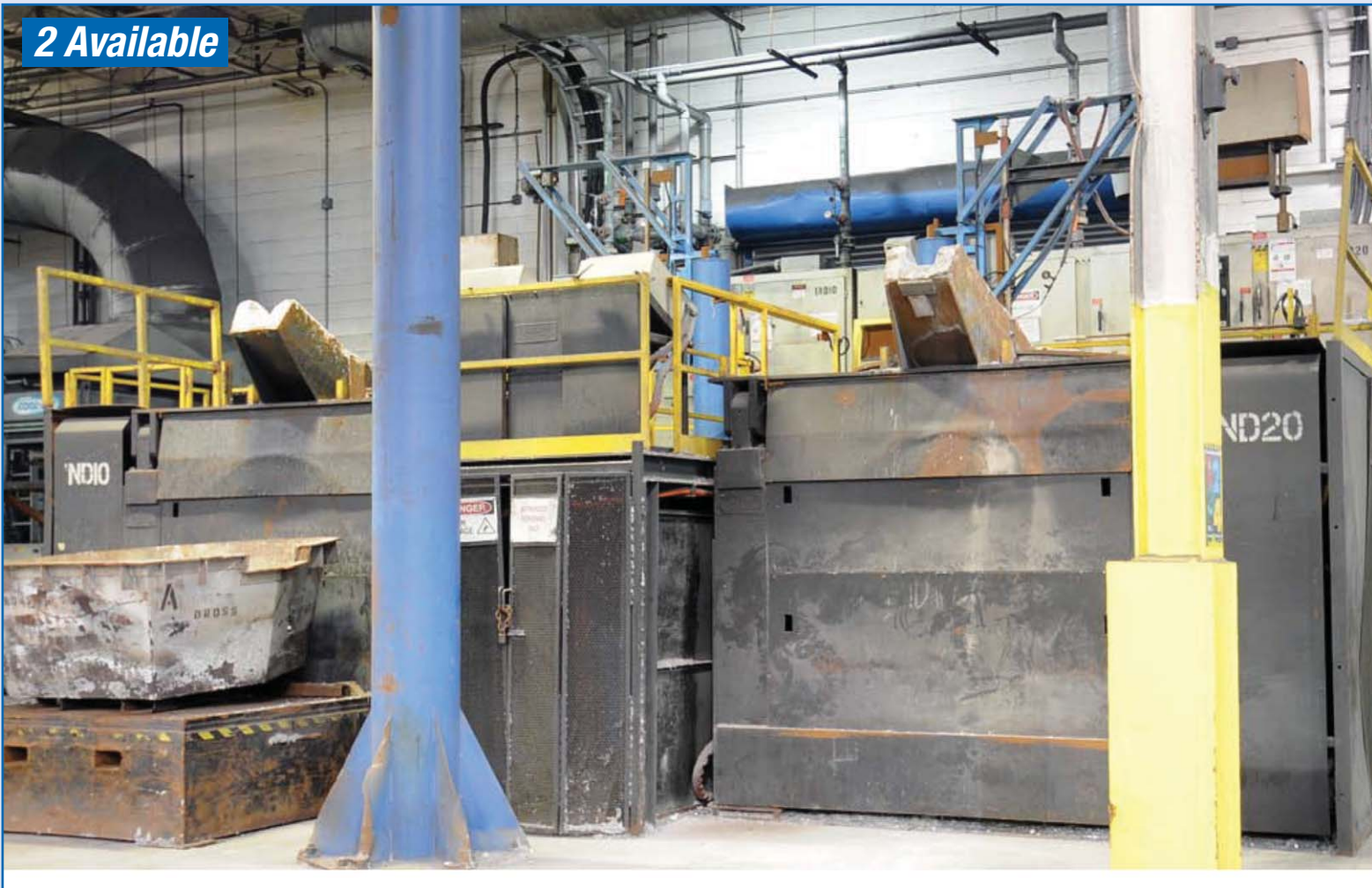
PARTIAL VIEW OF ABP CORELESS INDUCTION MELTING FURNACES
