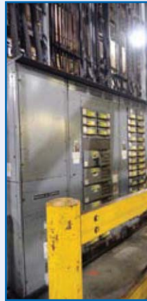
PARTIAL VIEW OF ELECTRICAL PANELS
