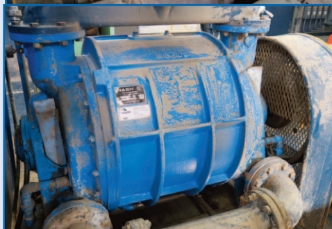
PARTIAL VIEW OF NASH VACUUM PUMPS
