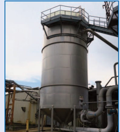
S1500 TCR 15,5P CLARIFIER
