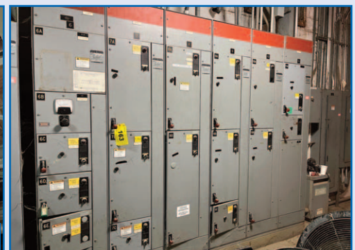
PARTIAL VIEW OF GE, CUTLER HAMMER MCC'S
