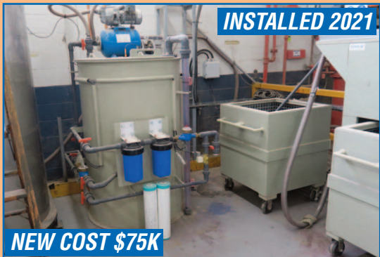
NISKAЕ WASTEWATER TREATMENT SYSTEM
