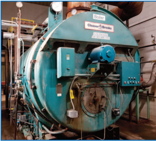
CLEAVER BROOKS CB 700-700 BOILER
