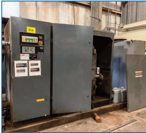
ATLAS COPCO GA90 COMPRESSOR
